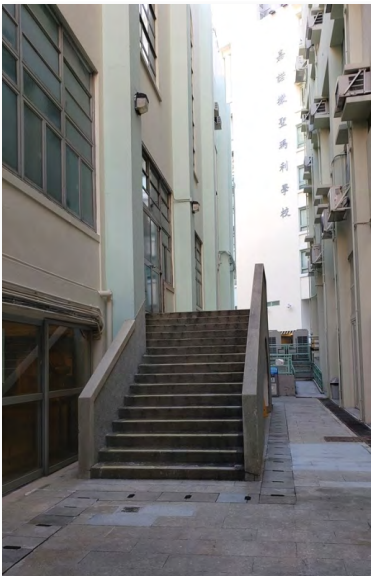
The lift for the School Hall Building will replace half of the arch staircase outside the Tuck Shop.
