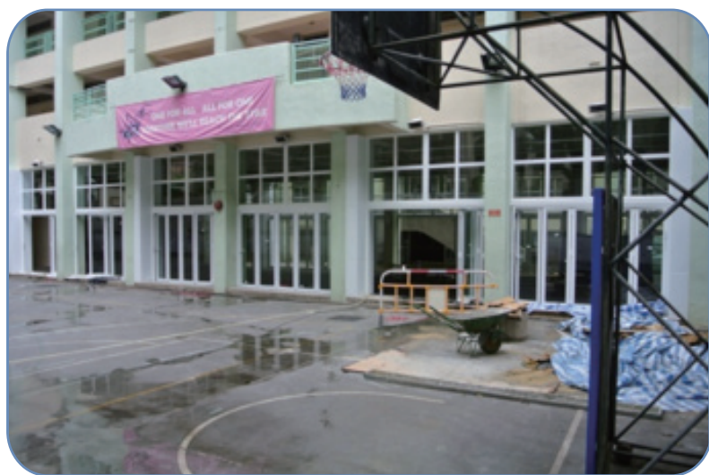
Folding glass doors being installed to enclose the covered playground at the ground level of the Magdalene Building.
